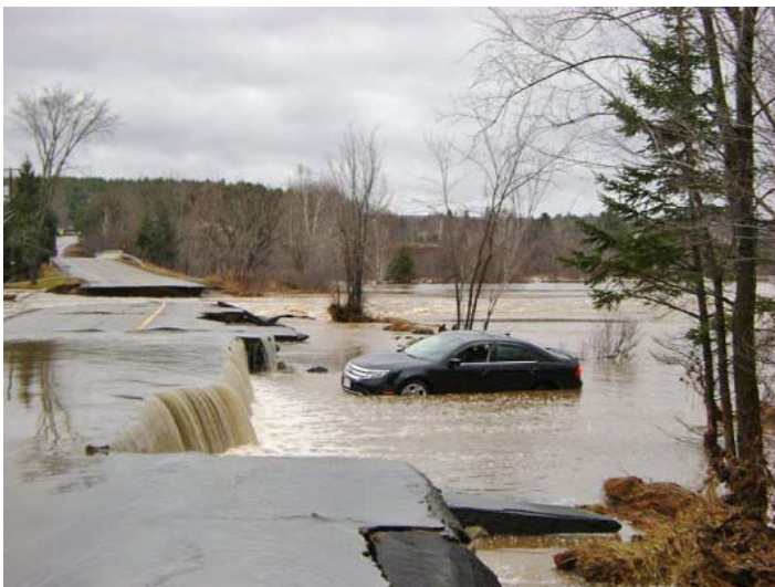
Road infrastructure damage due to flooding, Dec 2010.
